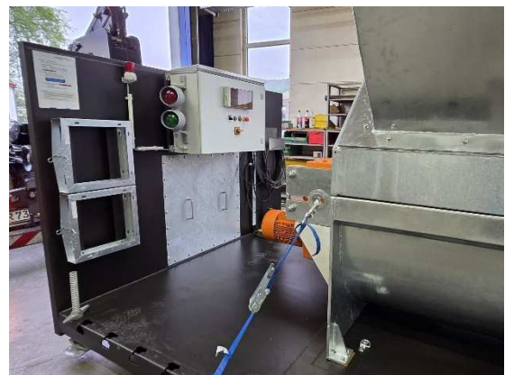
Control cabinet with plc and traffic light system
