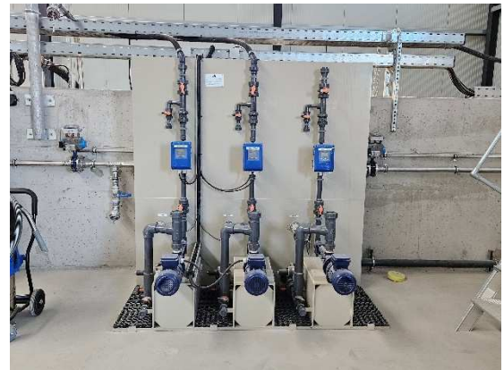
Flocculating agents dosing station
