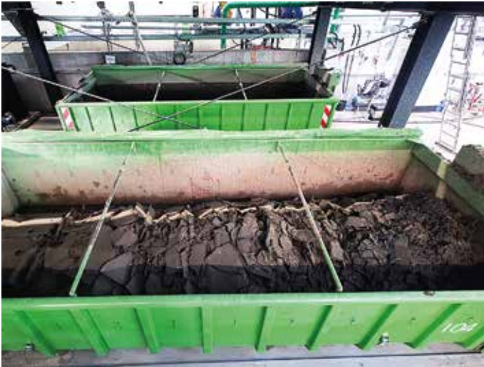
Filterkuchen in Container
