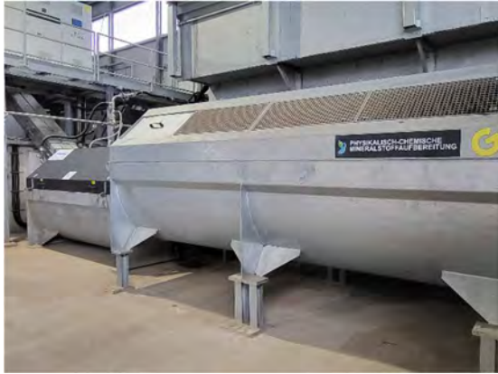
Dosing buffer (right) with recycling system (left)
