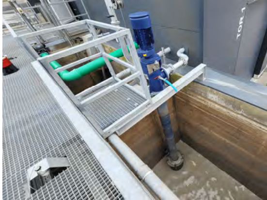
Agitator tank with feed pump centrifuge
