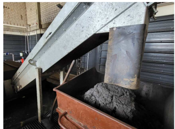
Mineral components from recycling machine
