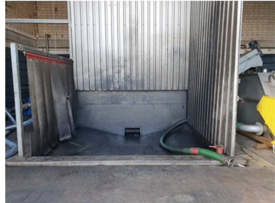
Receiving hopper for waste
