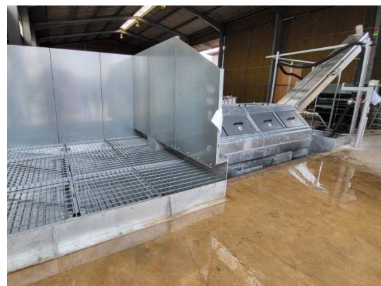
Final situation: Recycling system with material discharge
